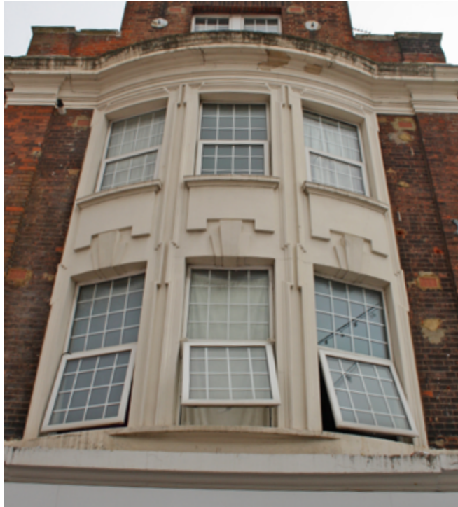
Inensitive replacement of traditional windows with uPVC units is harming the appearance of the conservation area.
