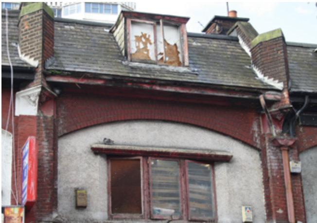
This building is in an extremely dilapidated condition due to lack of maintenance.
